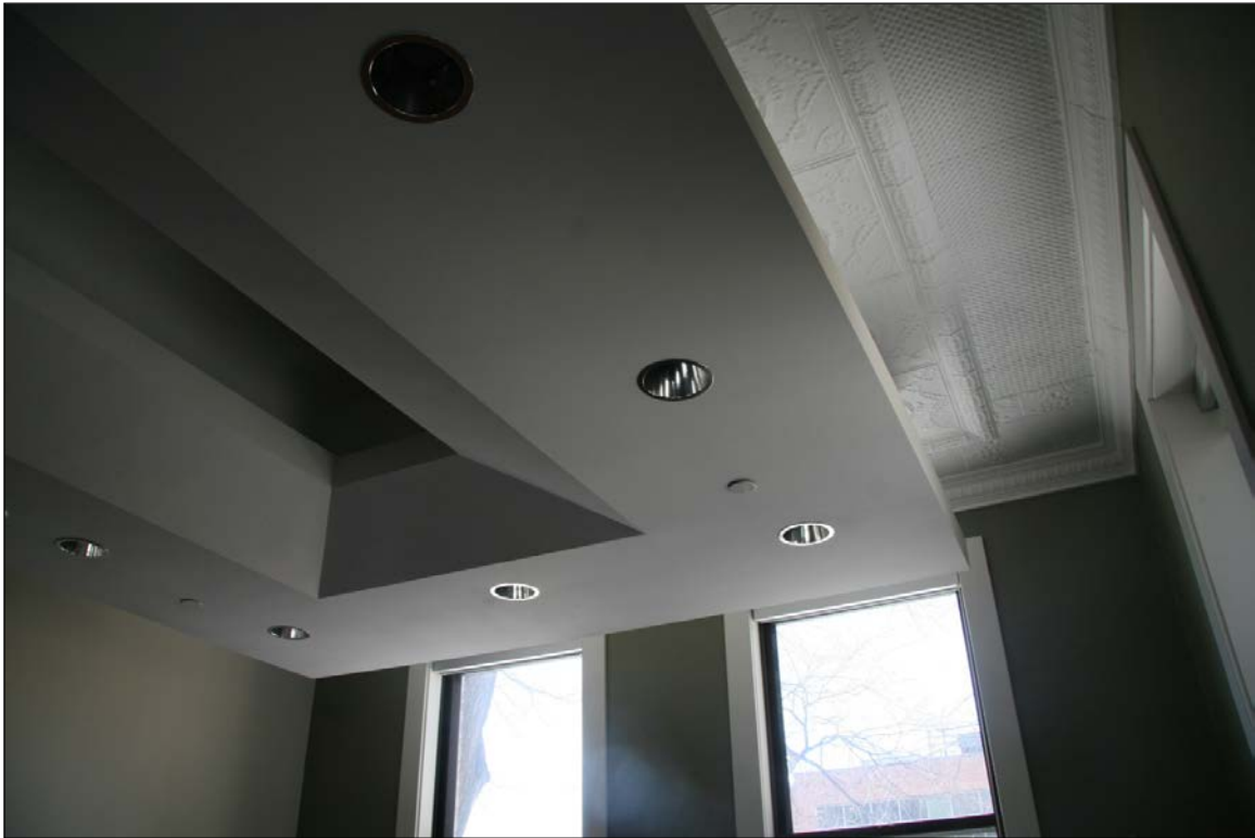
Plate 16 – Manitoba Medical College (University of Manitoba Faculty of Medicine Building), 750 Bannatyne Avenue, 2 nd floor classroom, 1913 addition with original tin ceiling exposed and repaired, 2018. ( T. Andreoglou, 2018. )
