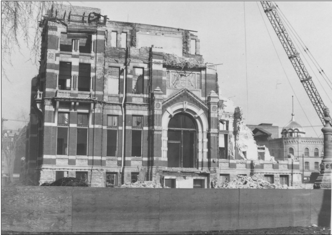
Plate 8 – Demolition of old City Hall continues, the bust of Queen Victoria still stands in its original location, 1962. ( City of Winnipeg Archives, i01473. )
