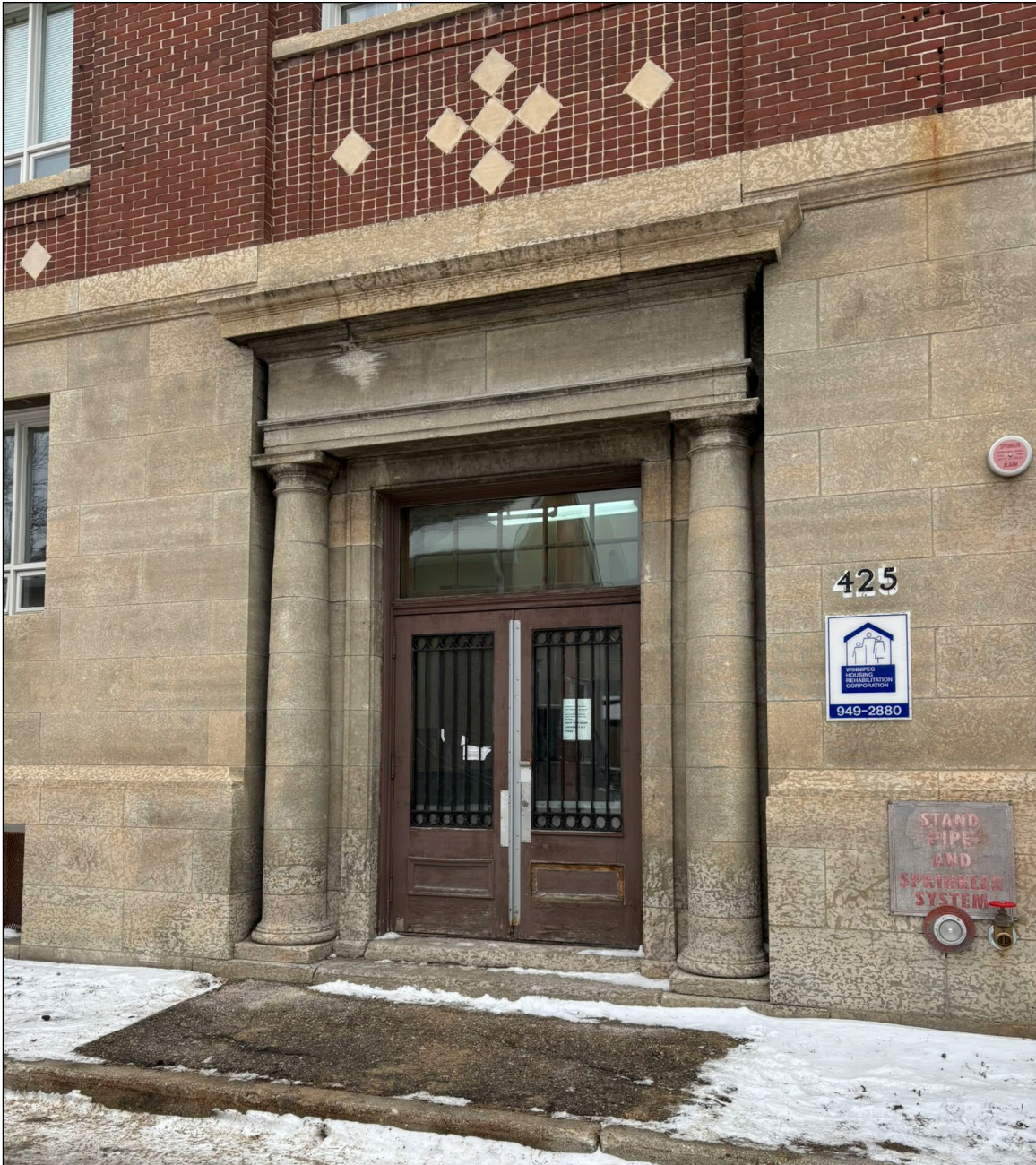
Plate 5 – Turner & Walker Block, 425 Henry Avenue, original main entrance, south façade, 2024. (M. Peterson, 2024.)
