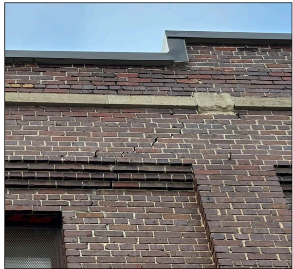
Plate 35 – Midland Railway Building, 200 Isabel Street, façade cracking, 2024. (M. Peterson, 2024 .)
