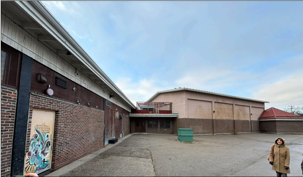
Plate 11 – Midland Railway Building, 200 Isabel Street, north façade and 1991 gymnasium addition, 2024. (M. Peterson, 2024.)
