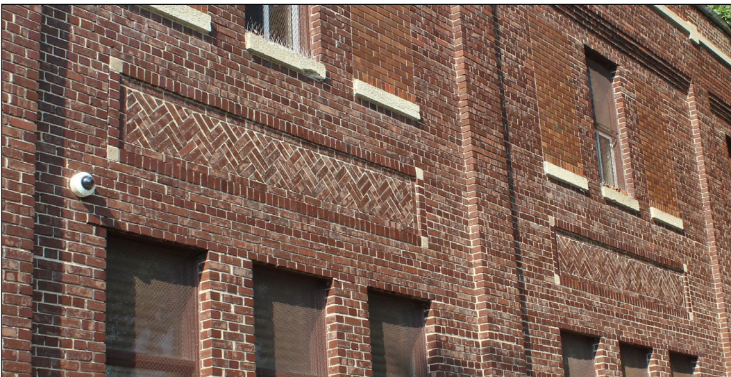
Plate 15 – Midland Railway Building, 200 Isabel Street, close up of spandrels, north façade, 2021. (M. Peterson, 2021.)
