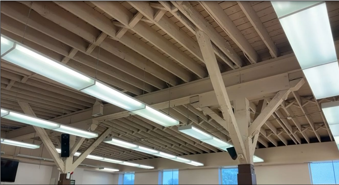
Plate 36 – Midland Railway Building, 200 Isabel Street, Central Community Centre, Unit 6, steel I-beam support, 2024. (M. Peterson, 2024.)
