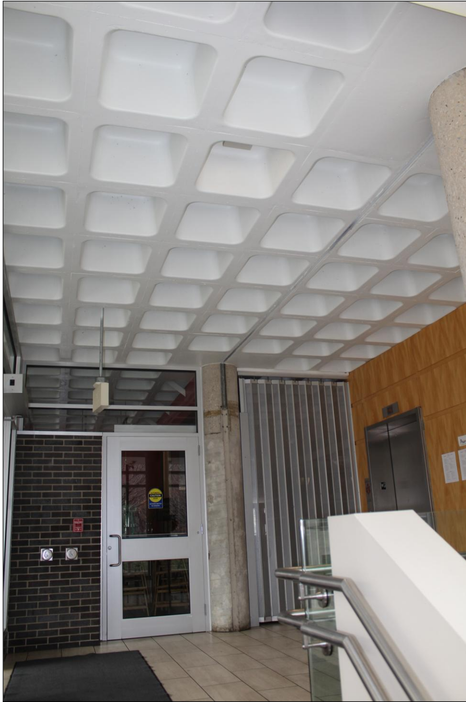
Plate 37 – Peguis Pavilion, Kildonan Park, 2015 Main Street, southeast corner entrance lobby with new door, partitioning and elevator, 2022. ( M. Peterson, 2022. )
