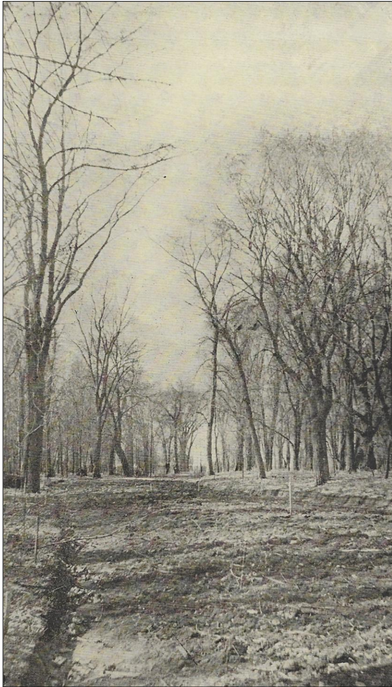
Plate 3 – Road grading at Kildonan Park, 1910. ( Winnipeg Public Parks Board, Annual Report, 1910, p. 28. )
