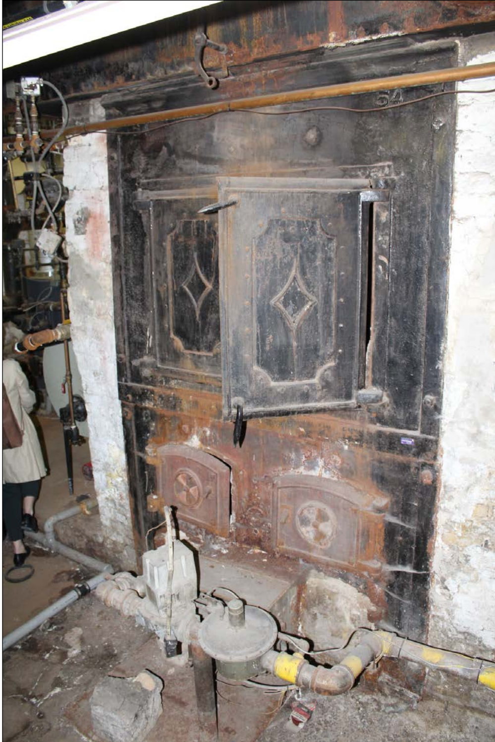
Plate 19 – McLaren Hotel, 554 Main Street, decommissioned boiler in basement, 2019. ( M. Peterson, 2019. )
