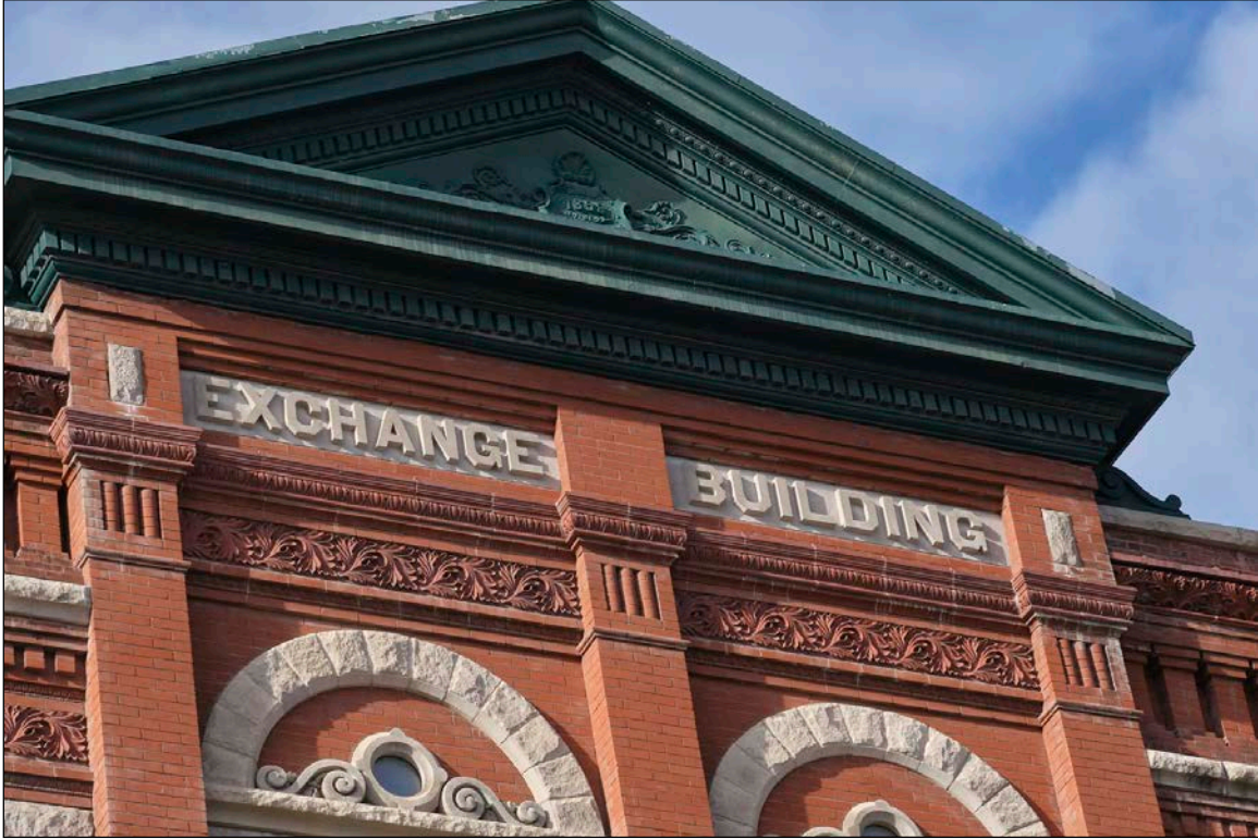
Plate 14 – Exchange Building, 160 Princess Street, fourth floor detail, front (east) façade, 2019. ( G. Cline, 2019. )
