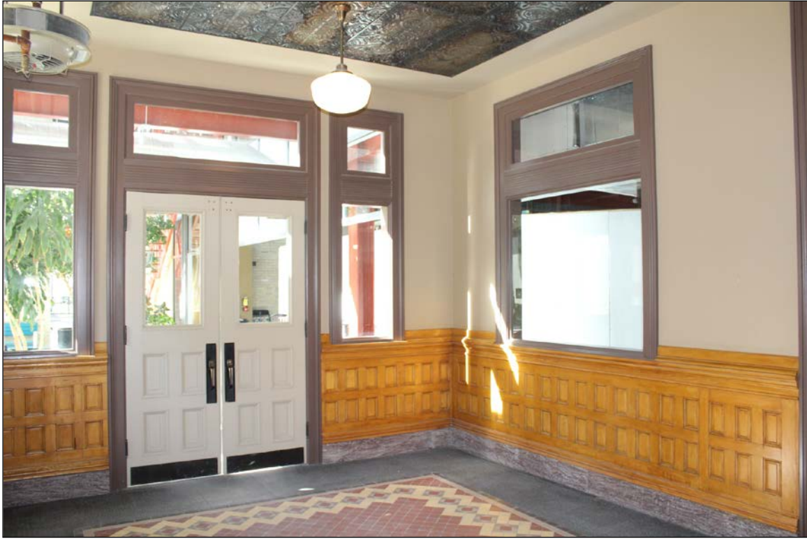
Plate 23 – Red River College Princess Street Campus, 140 Princess Street, rebuilt entrance foyer of 160 Princess Street with oak wainscoting, marble border and baseboards and tile floor, 2019. The tile floor was relocated from the original third floor. (M. Peterson, 2019.)
