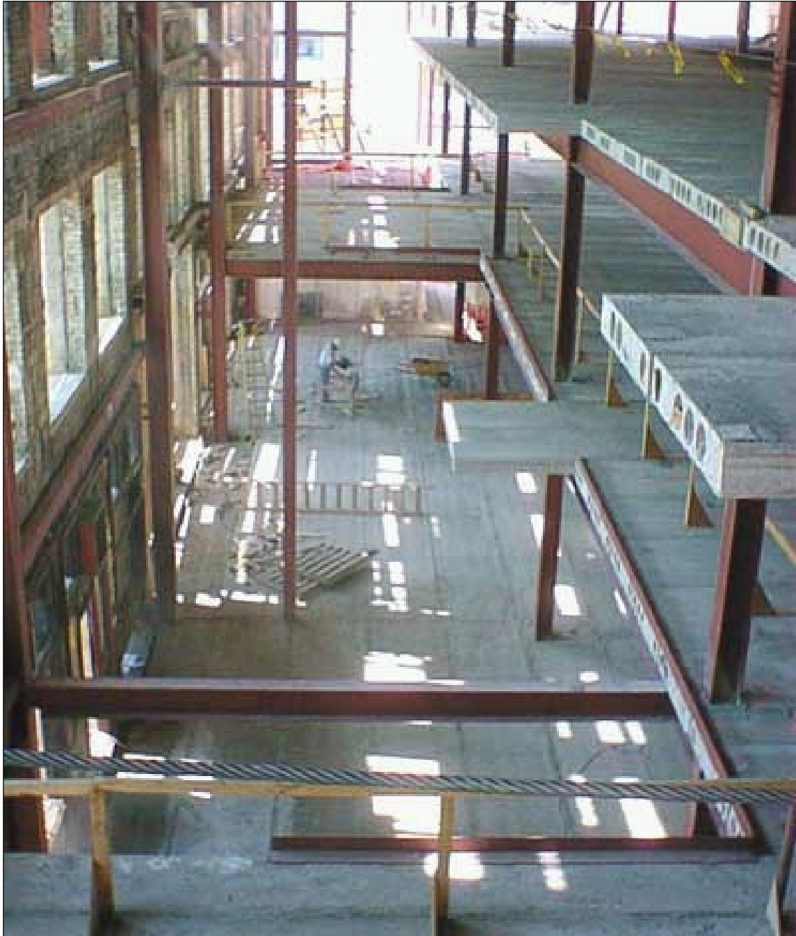
Plate 21 – Red River College Princess Street Campus, 140 Princess Street, construction of new building, rear (west) façade, 2001. ( M. Peterson, 2001. )
