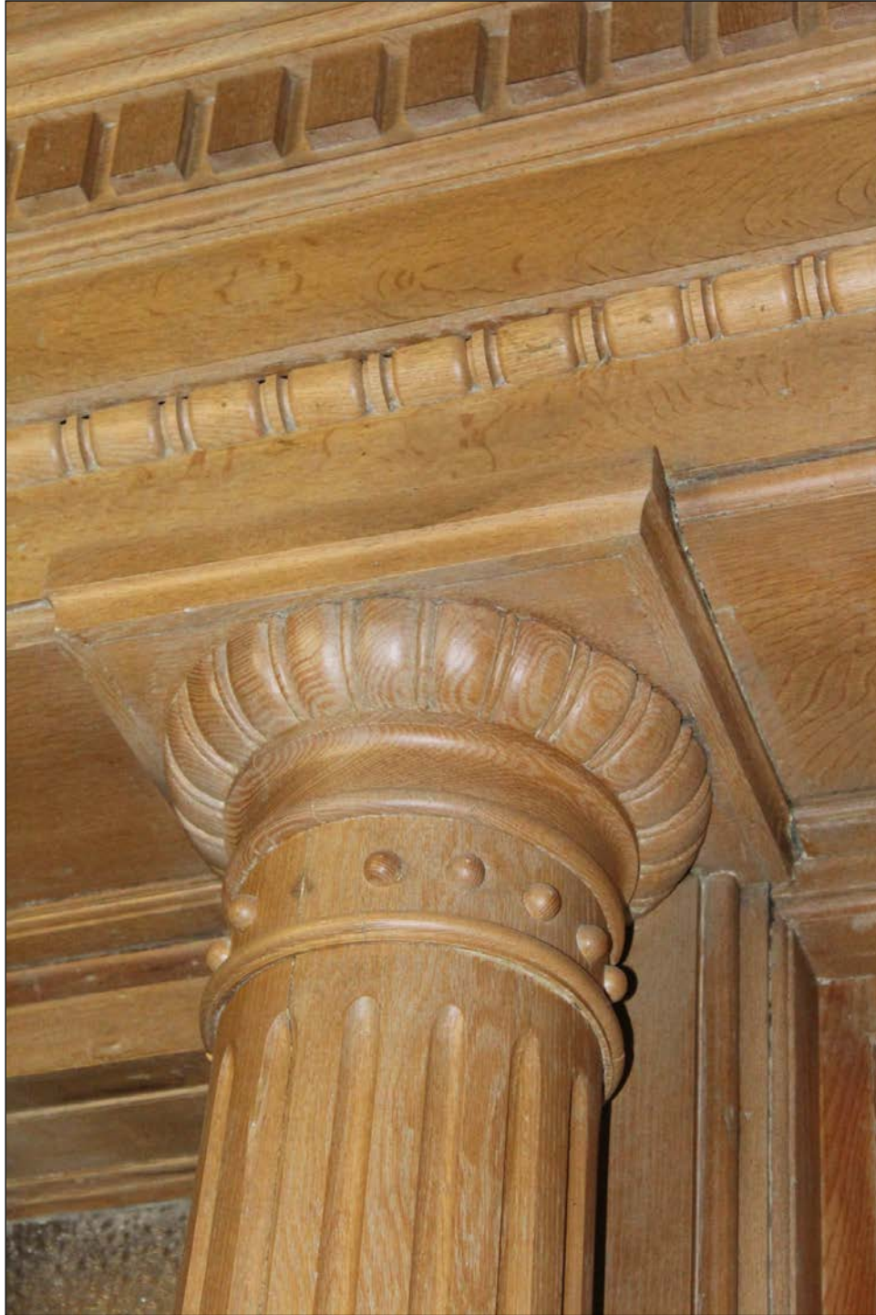
Plate 28 – Red River College Princess Street Campus, 140 Princess Street, original 160 Princess Street third floor oak detailing rebuilt in its original location, 2019. ( M. Peterson, 2019. )
