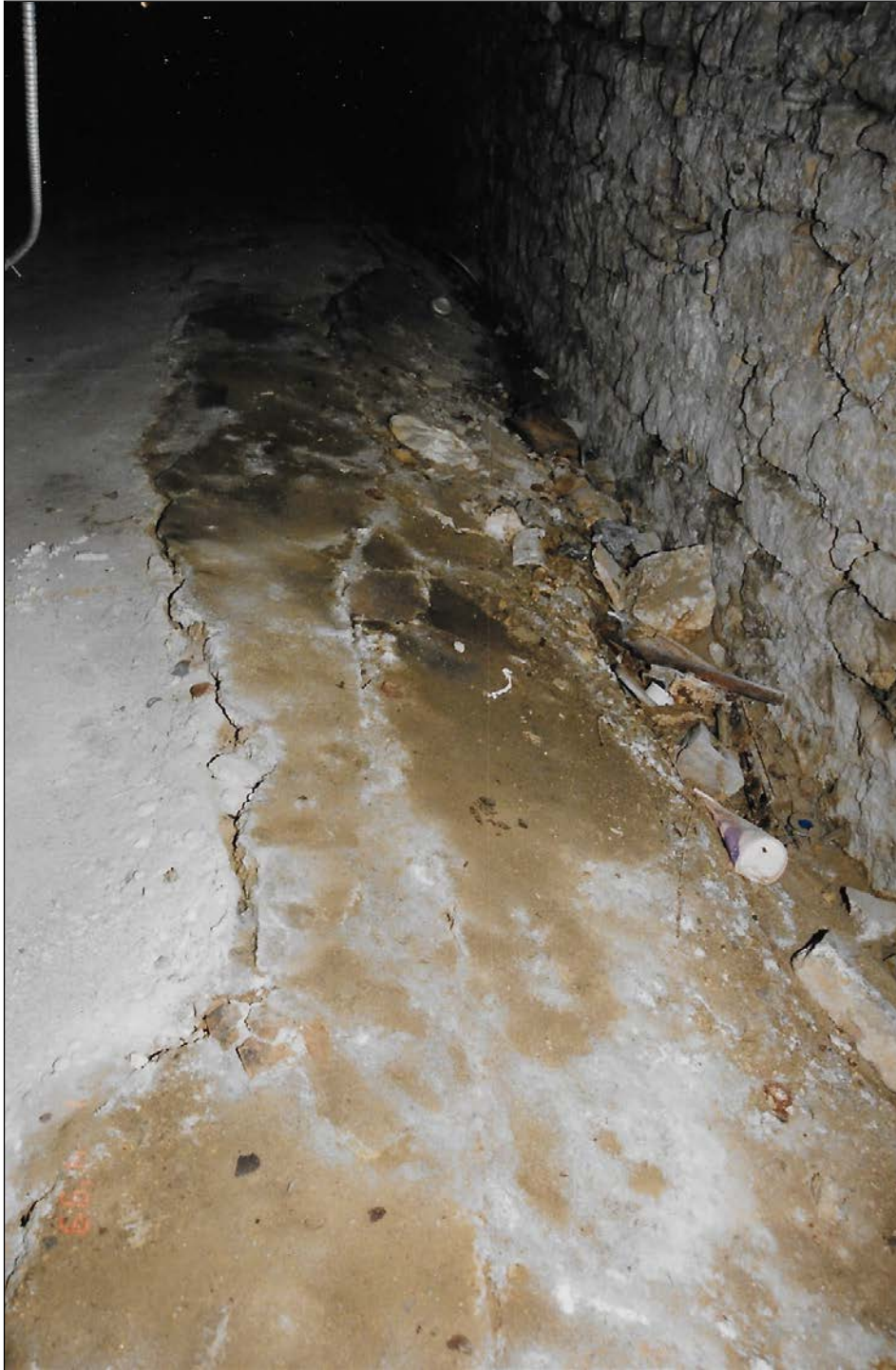
Plate 11 – Utility Building, 164 Princess Street, north wall settlement and slab heave, 1999. ( Eschmade, 1999, Image #75. )
