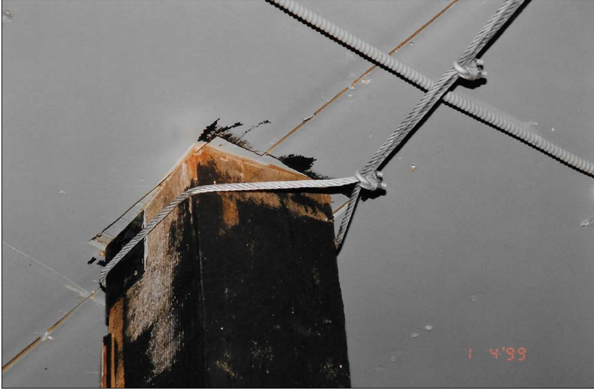
Plate 12 – Utility Building, 164 Princess Street, cable tie to support north wall, 1999. ( Eschmade, 1999, Image #73. )
