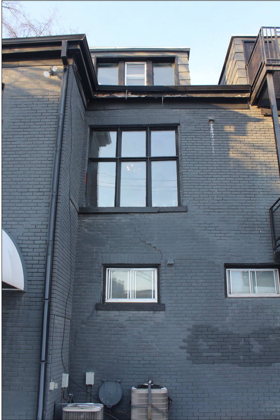
Plate 4 – John C. Falls House, 36 Roslyn Road, brick movement, rear (south) façade, 2021. ( M. Peterson, 2021. )
