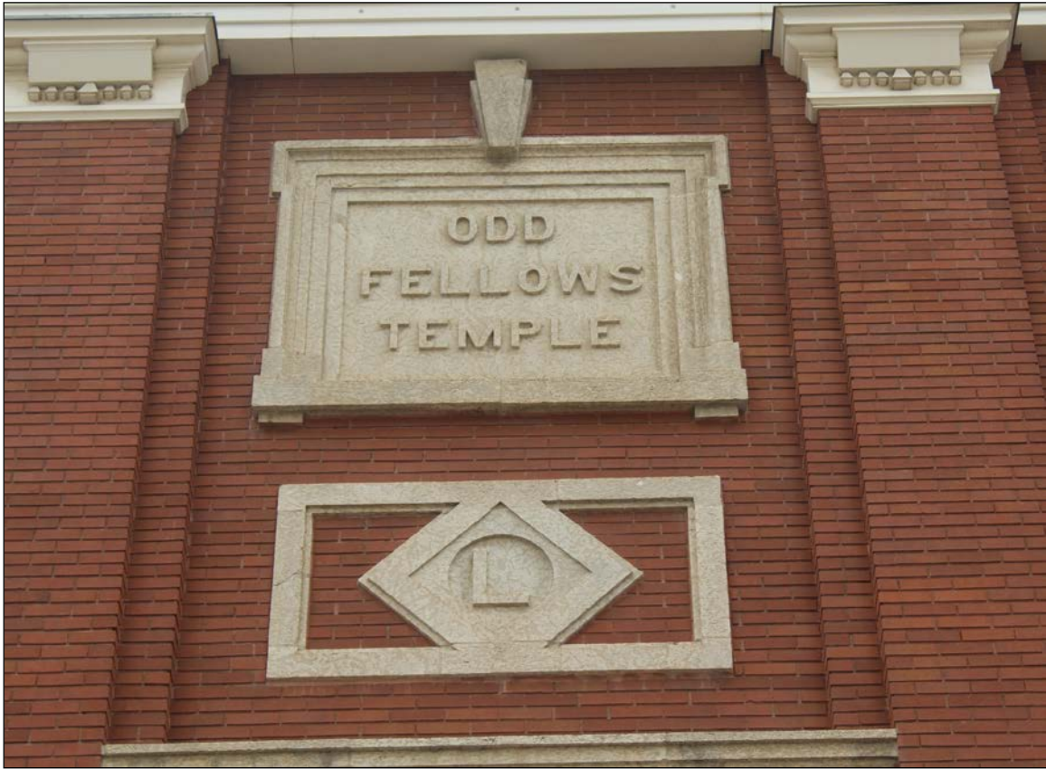
Plate 7 – Independent Order of Odd Fellows Temple façade, 0 The Promenade, detail of front façade, 2020. ( M. Peterson, 2020. )
